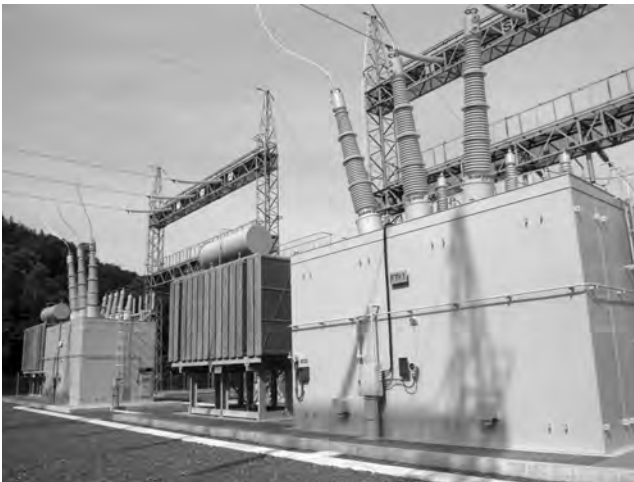
Fig. 7 70MVA Roof-Delta Connection Transformer This figure shows an outside view of the 70MVA roof-delta connection transformer. The primary side is 220kV and the secondary side is 60kV × 2 lines.
