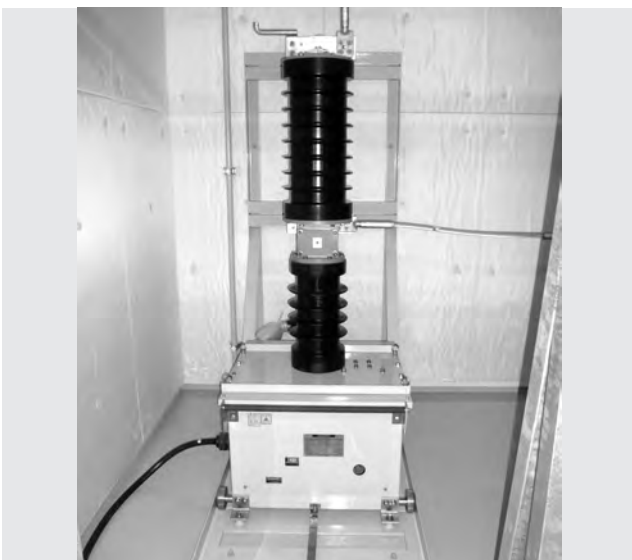
Fig. 10 36kV Changeover Switch
