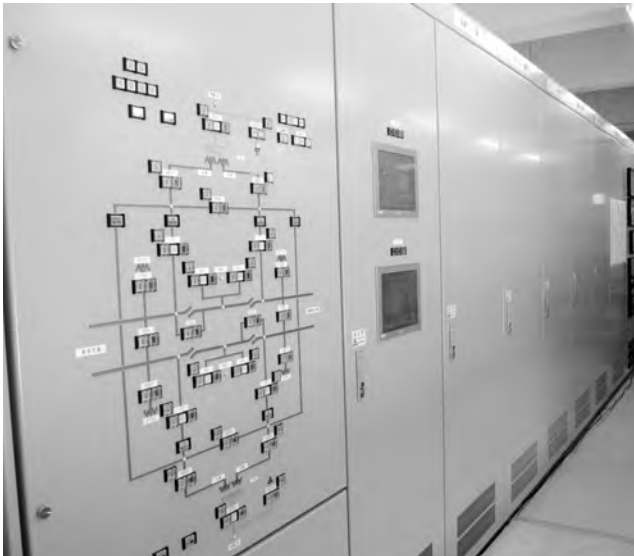
Fig. 14 Monitoring and Control Panel at Shin-Gyokuto SS
