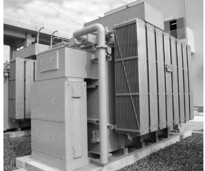
Fig. 8 20MVA Scalene Scott-Connection Transformer This figure shows an outside view of the 20MVA scalene Scott-connection transformer. The primary side is 66kV and the secondary side is 30kV.
