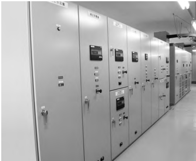
Fig. 16 High Voltage Control Panel of Shin-Omuta DP This figure shows an outside view of the high voltage control panel of Shin-Omuta DP. Cost reduction by use of air insulation and self-cooling method is realized.
