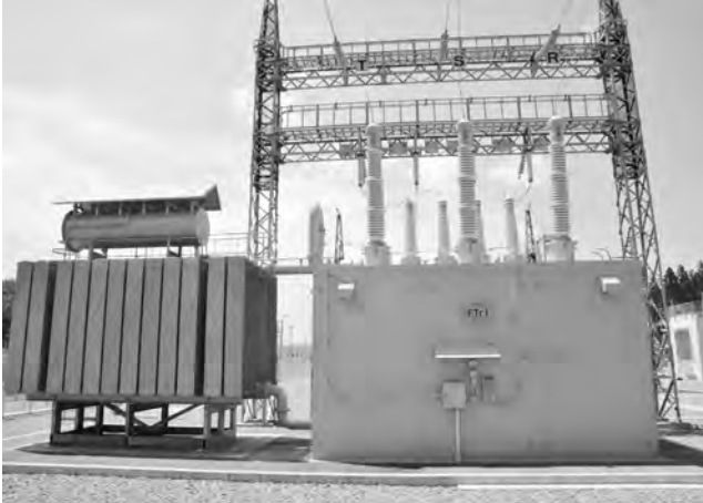
Fig. 6 50MVA Scott-Connection Transformer This figure shows an external view of the 50MVA Scott-connection transformer. The primary side is 154kV and the secondary side is 60kV × 2 lines.
