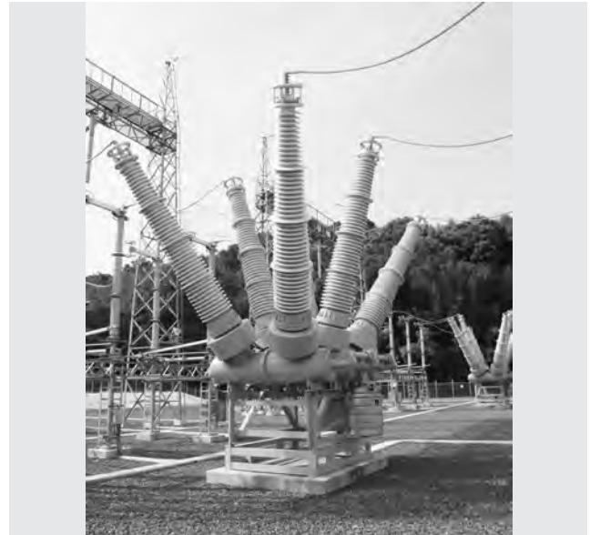
Fig. 5 240kV Gas Circuit-Breaker
