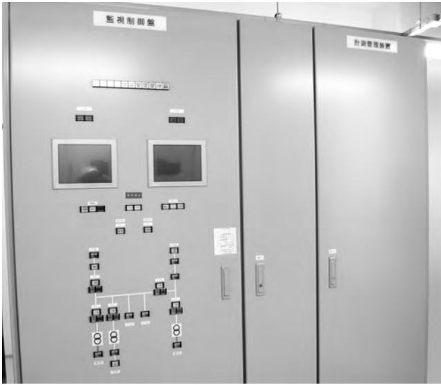
Fig. 19 Monitoring and Control Panel of Shin-Omuta DP
