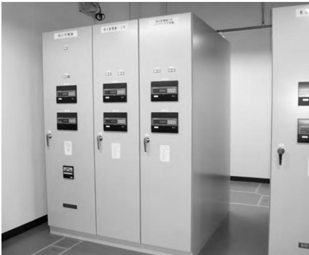
Fig. 17 Dry Air Circuit-Breaker of Kanahama DP This figure shows an outside view of the high voltage control panel of Kanahama DP. Dry air insulation is employed, which affects the environment less, and maintenance is easy.
