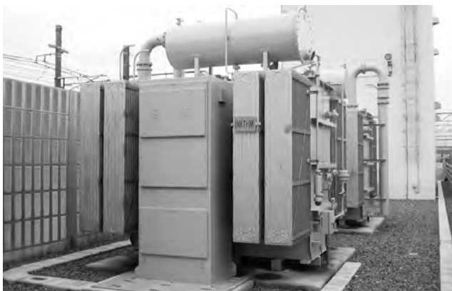
Fig. 3 Interconnected Transformer Group
