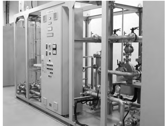
Fig. 4 Inverter Panel and Cooling Pump
