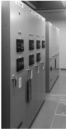
Fig. 13 Medium-Voltage Switchgear at the Nishi-Kasahara DP
