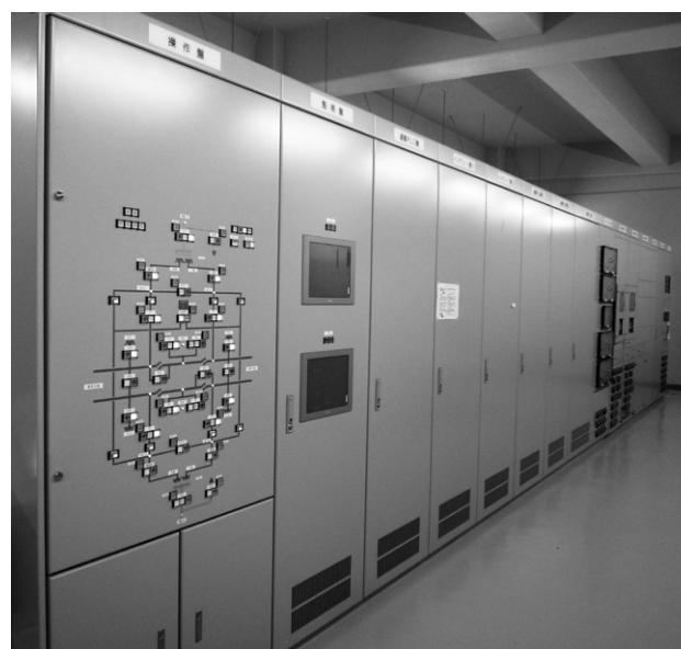
Fig. 7 Monitoring and Control Panel for the Shin-Kurobe SS
