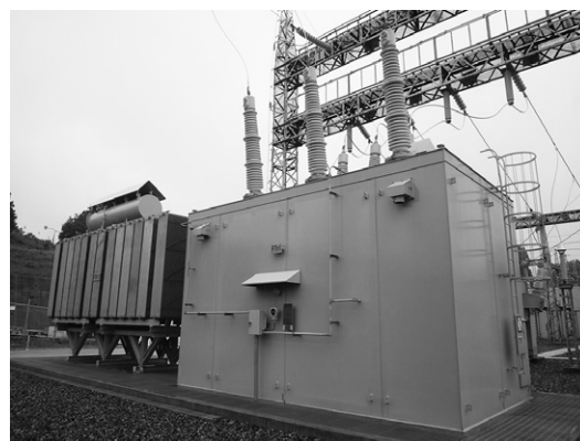
Fig. 4 70MVA Scott-Connection Transformer
