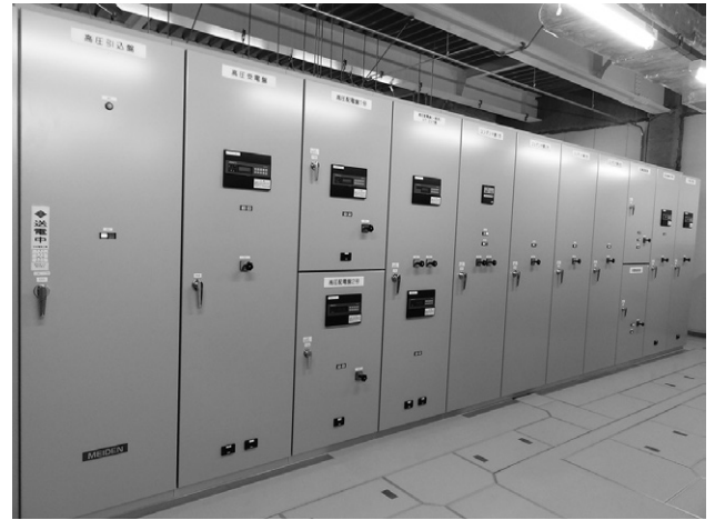
Fig. 14 Medium-Voltage Switchgear at the Itoigawa DP
