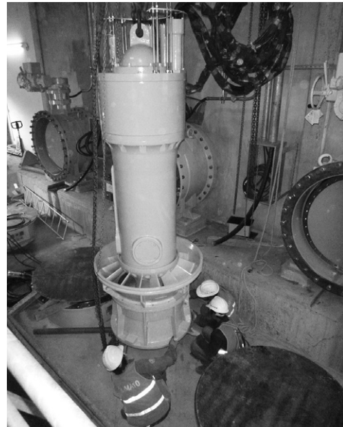
Fig. 2 150kW Permanent Magnet Sub-Water Turbine Generator
