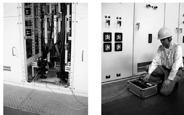
(b) Testing by using the artificial ground fault tester
