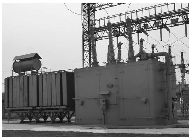
Fig. 6 Roof-Delta Connected Transformer
