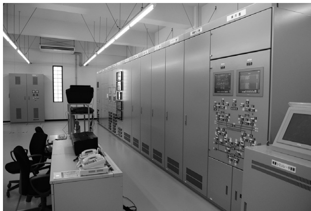
Fig. 11 Supervisory Control Panels for Shin-Hakodate Substation
