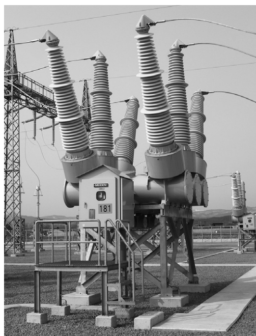
Fig. 3 Power Receiving VCB
