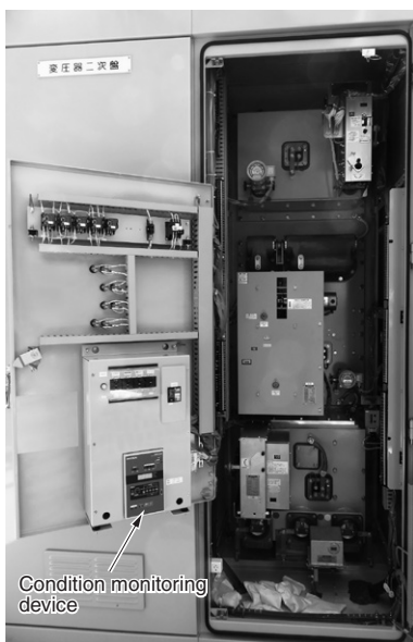
Fig. 2 Condition Monitoring Device Installed in the C-GIS
