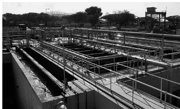
Fig. 1 Industrial Used Water Treatment Facility
