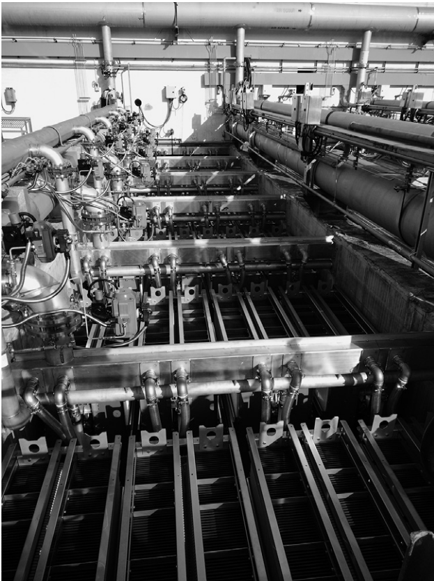
Fig. 7 Ceramic MF System at the Chestnut Avenue Water Works
