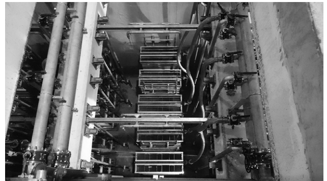
Fig. 5 MBR System at the Changi Water Reclamation Plant
