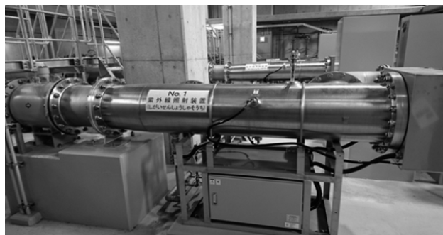
Fig. 3 Ultraviolet Ray Treatment Facility at the Watarase Drinking Water Treatment Plant
