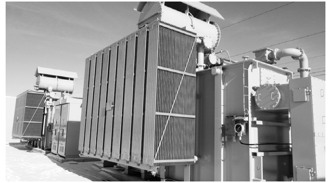
Fig. 3 Traction Power Transformer
