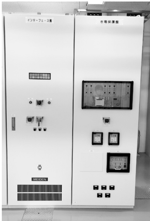
Fig. 7 Power Distribution Board
